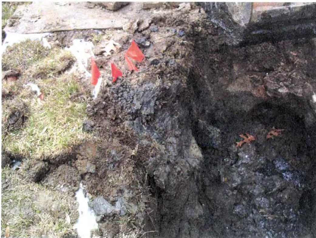
Picture 2: UST 398Acorn tank pit with soil staining.
